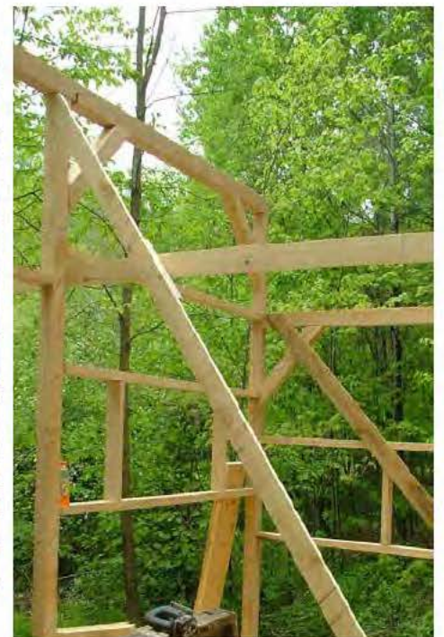
Figure 7. Brace your front wall in the center, over the door, not to interfere with the loft.
